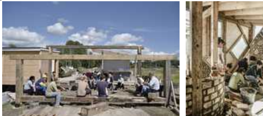
Photo 7+8: A break with trainees and farmers during the assembly of the timber structure and workshop participants laying the cordwood-floor.
