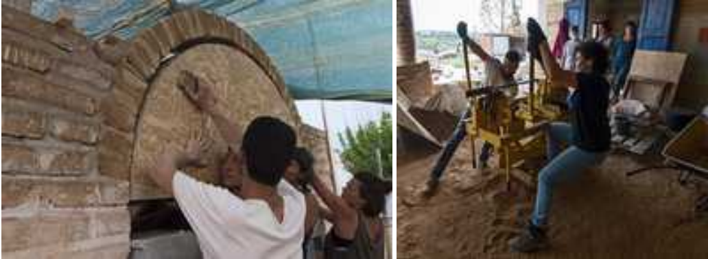
Photo 1+2: Trainees on the building site and while pressing CEB in Oficina's Raw earth laboratory.
