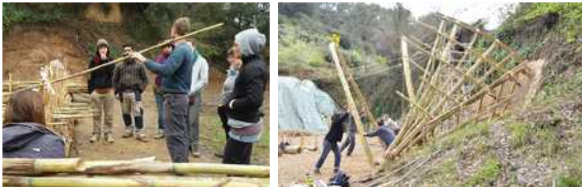
Photo 10 + 11: Learning the criteria to classify the harvested canes and erection of a structural cane arch.
