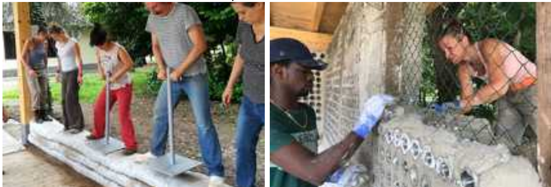
Photo 16 + 17: Fun and effort while compacting the super-adobe wall and collaboration of trainees with different cultural backgrounds on the bottle-wall.
